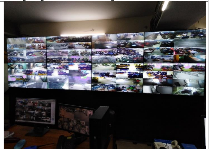
Central Monitoring and Surveillance Centre in the Building
