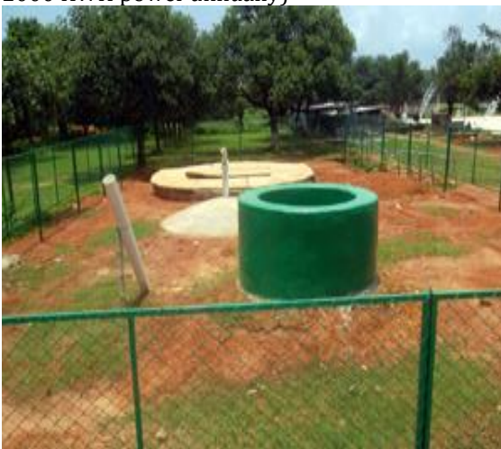
Example of Biogas plant (Daffodil International University)
