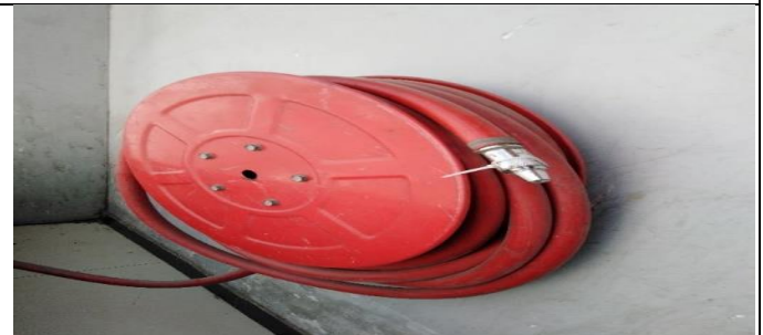
Firefighting tools in the building
