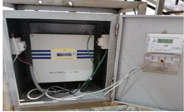
Solar panel energy grid
