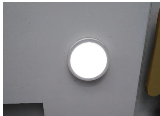
Sensor-based LED lighting system in the buildings
