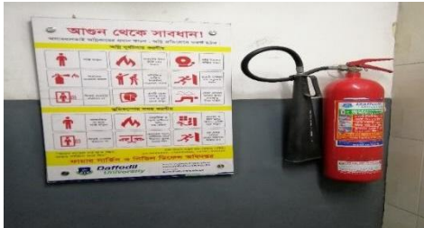
Fire Extinguisher along with Instructions to be followed (in local language) during fire and other accidents
