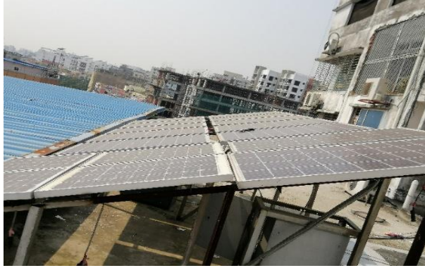
Campus rooftop Solar Panel used for using 1500 KWH power annually
