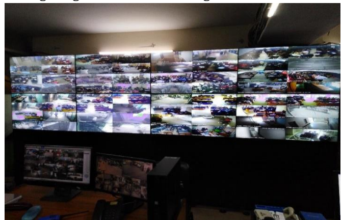
Central Monitoring and Surveillance Centre in the Building
