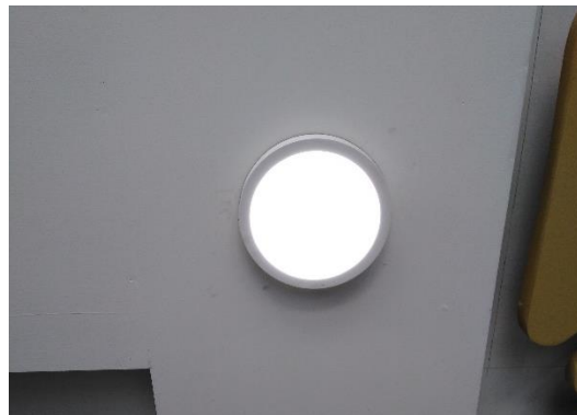
Sensor-based LED lighting system in the buildings
