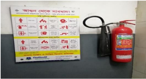
Fire Extinguisher along with Instructions to be followed (in local language) during fire and other accidents
